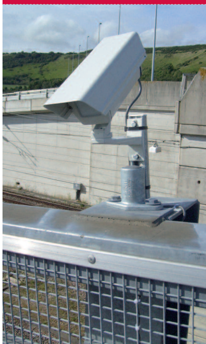
Campbell's new system is helping keep freight moving at the Eurotunnel terminal
