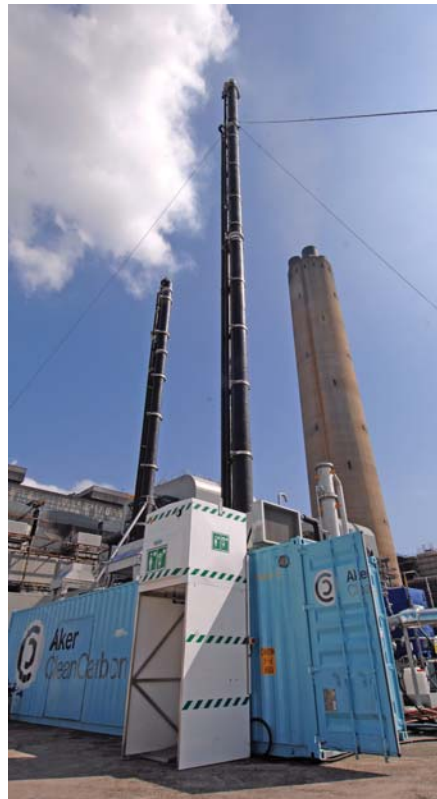
The UK's first slipstream capture plant on an operational coal-fired plant has been operating at Longannet, Scotland
